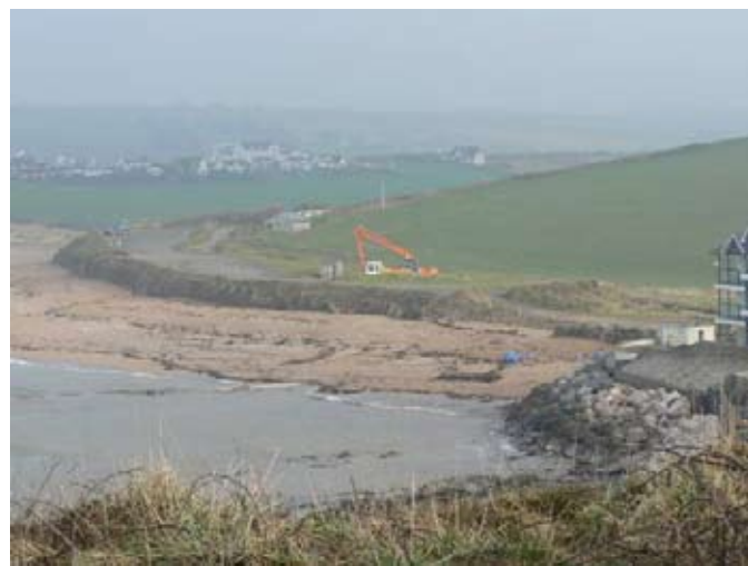
The car park area at the start of the project © Simon Hill, National Trust
